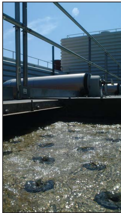
■ A comprehensive water treatment and tower maintenance program helps control the growth of Legionella in cooling towers. Photo courtesy of Ashland Water Technologies.
